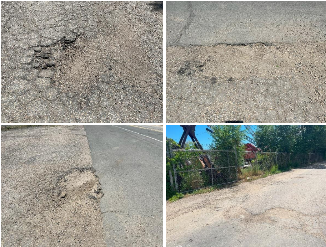
Figure 2. Poor Provisions or Unsafe Conditions for Vehicles
