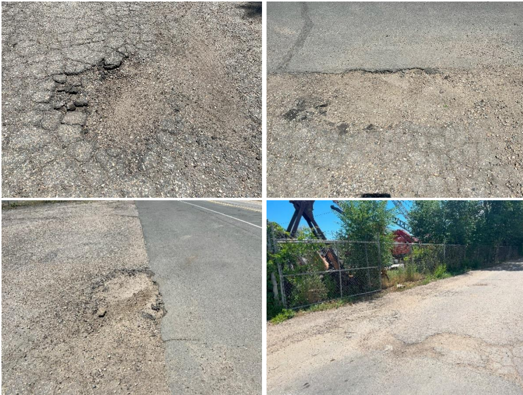
Figure 2. Poor Provisions or Unsafe Conditions for Vehicles
