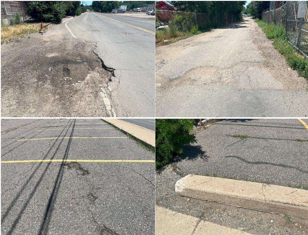
Figure 15. Deteriorated Pavement and Curbs
