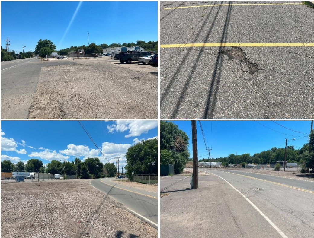
Figure 13. Deteriorated On-site Parking Surfaces, and Curb and Gutter
